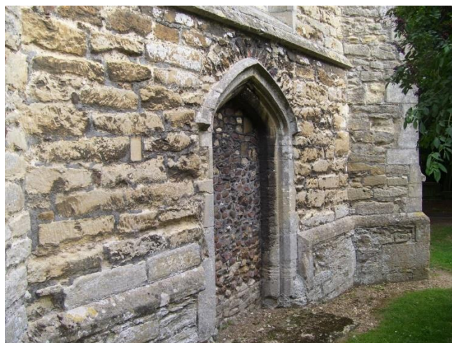
16 Blocked doorway at the West end of the Tower.
